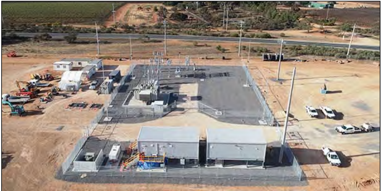
Figure 2-2: Typical substation and operations compound (ASLAT Consulting 2020: Figure 24)
